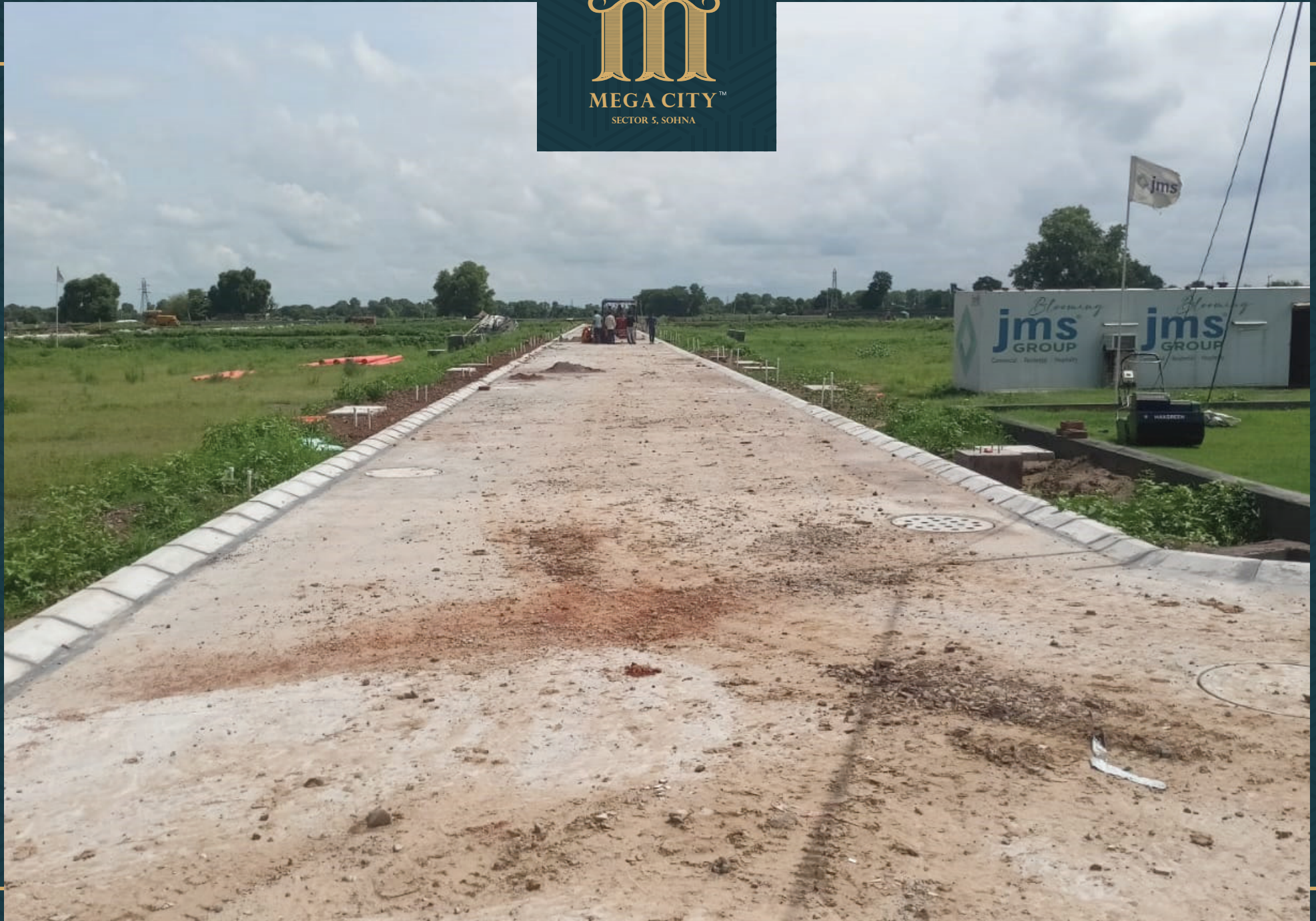
Road no 3 Water Supply, Sewerage, Road Trimix, Street Lights Foundation Completed, Road Side Footpath Work In Progress
