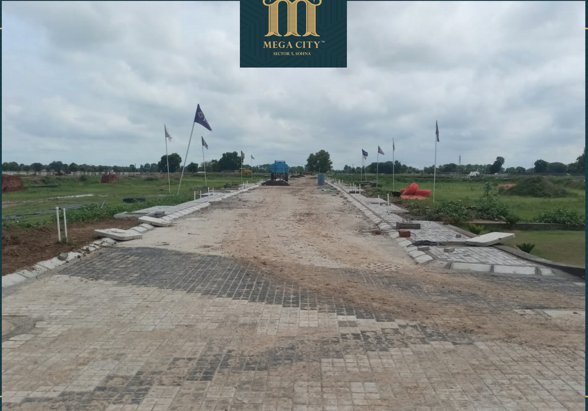
Road no 4 Water Supply, Sewerage, Road Trimix, Street Lights Foundation Completed Road Side Footpath Work In Progress
