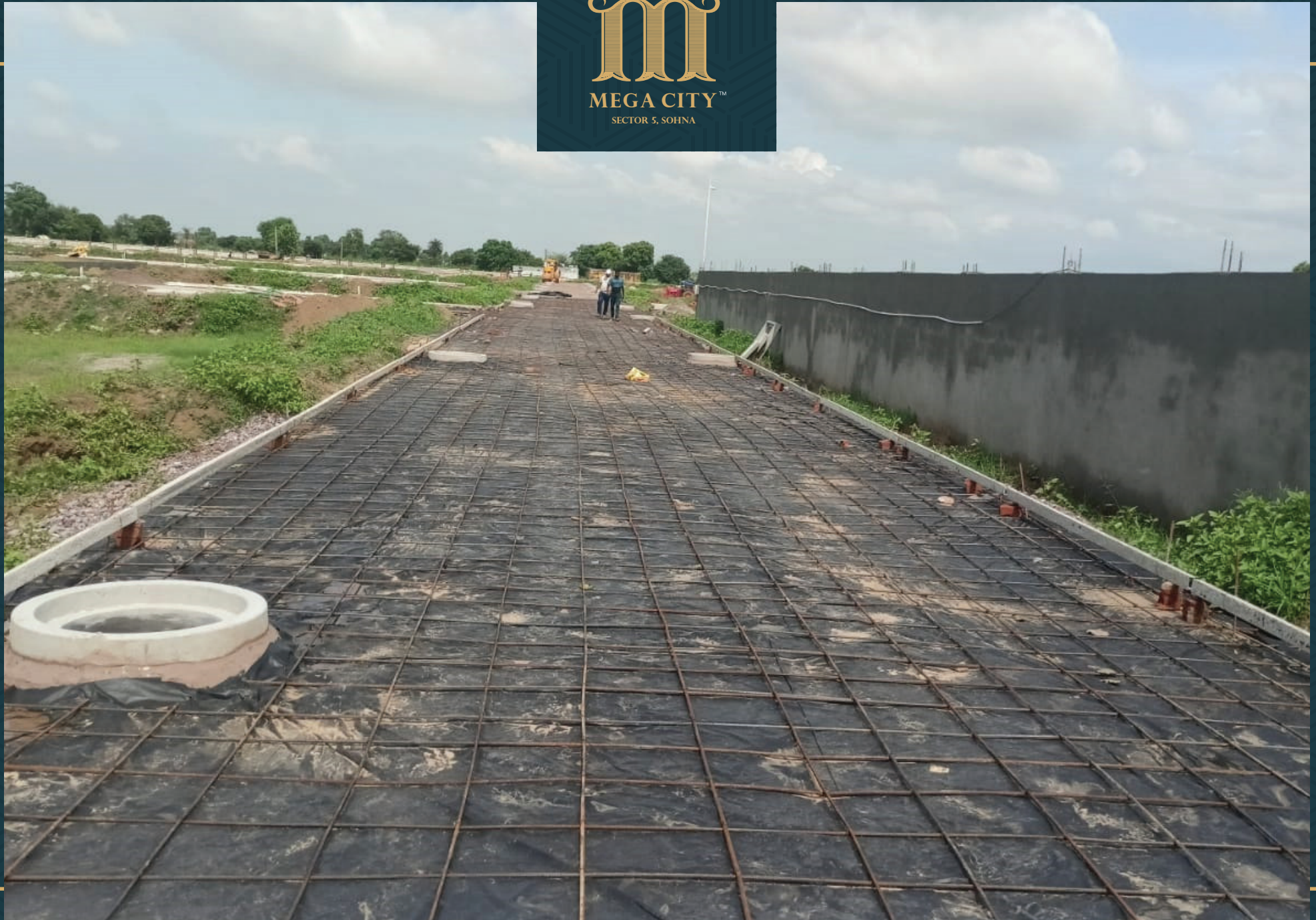
Water line, Sewerage Lines, Storm Water Lines and Road WMM Completed, Trimix Work in Progress
