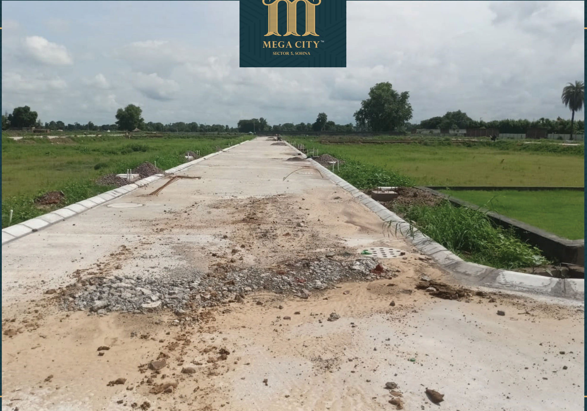
Road no 2 Water Supply, Sewerage, Road Trimix, Street Lights Foundation Completed, Road Side Footpath Work In Progress
