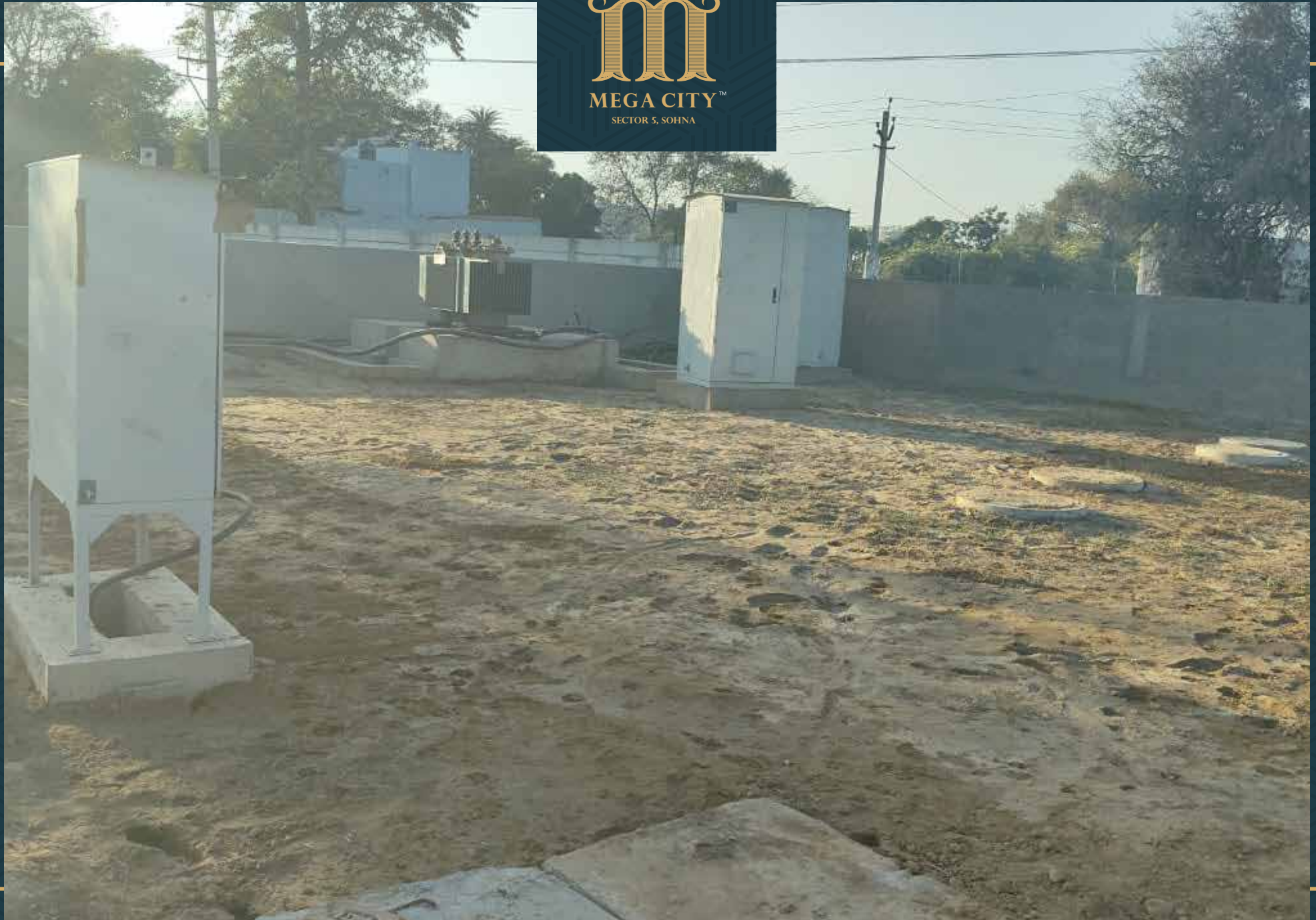
Electrical sub station equipment installation done and cable connection work in progress
