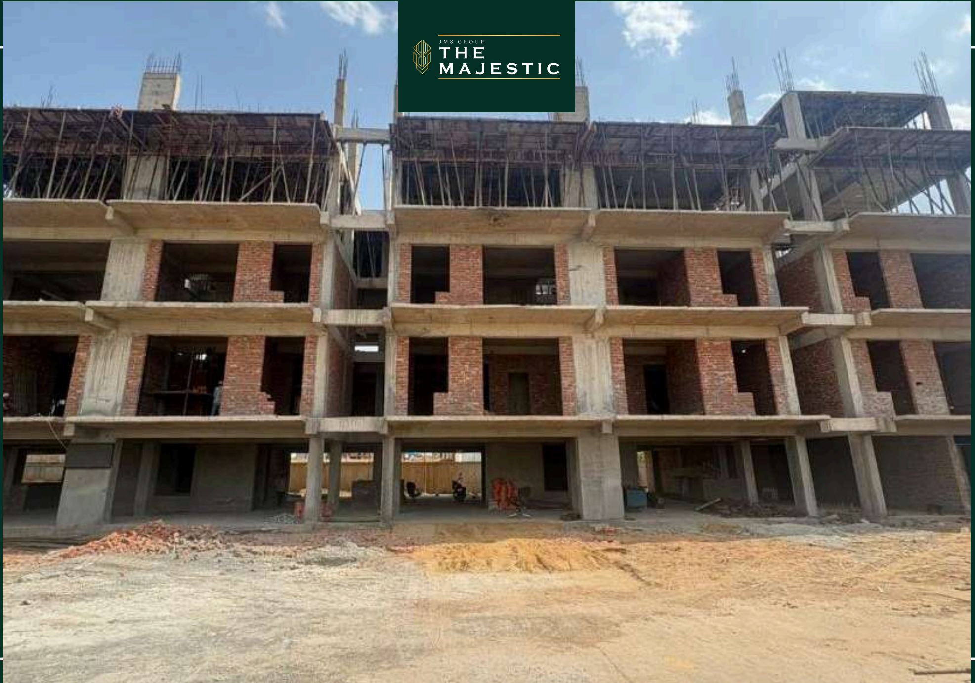
Plot 374-378 1st and 2nd floor brick work completed & top floor terrace shuttering work in progress
