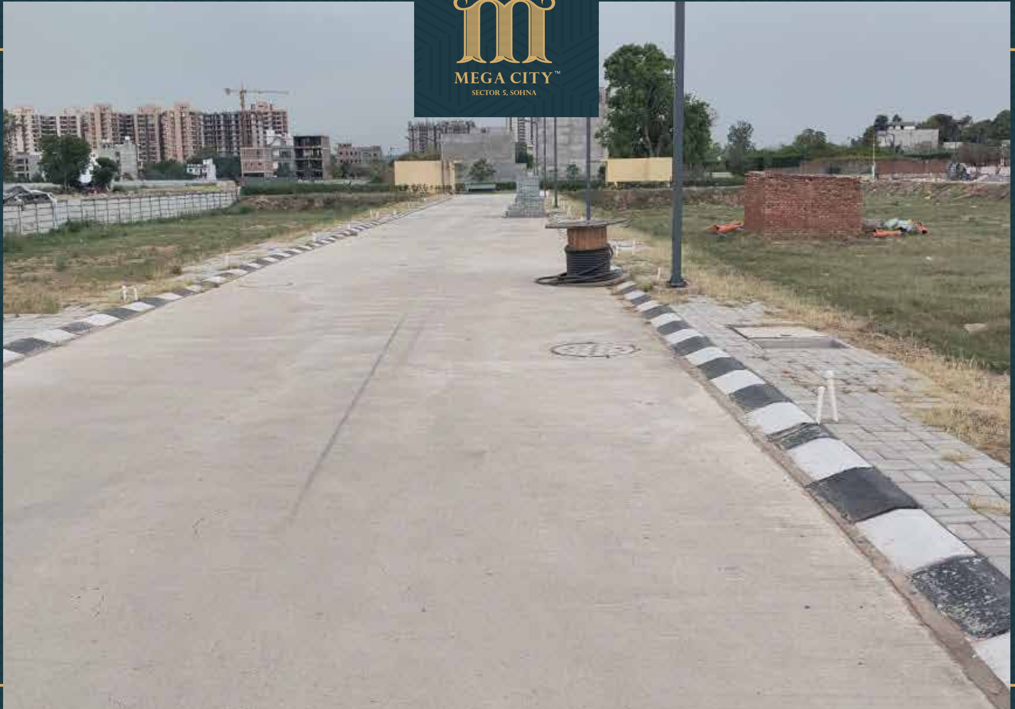
Road no. 8 development work completed including electrical cable lines. Plantation work in progress
