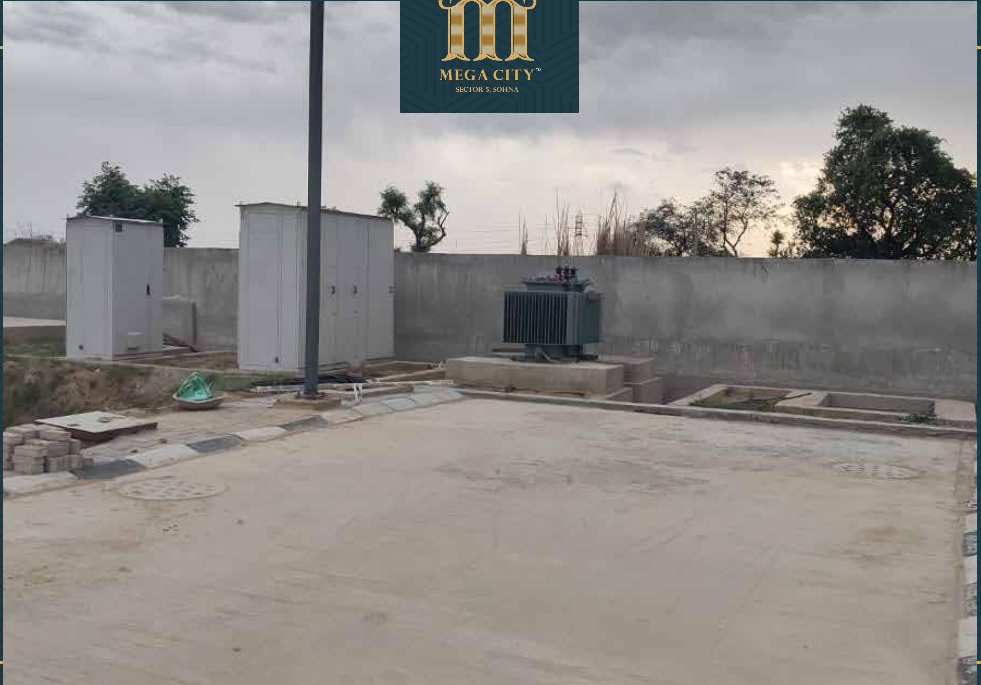
Electrical sub station 3 equipment installation done
