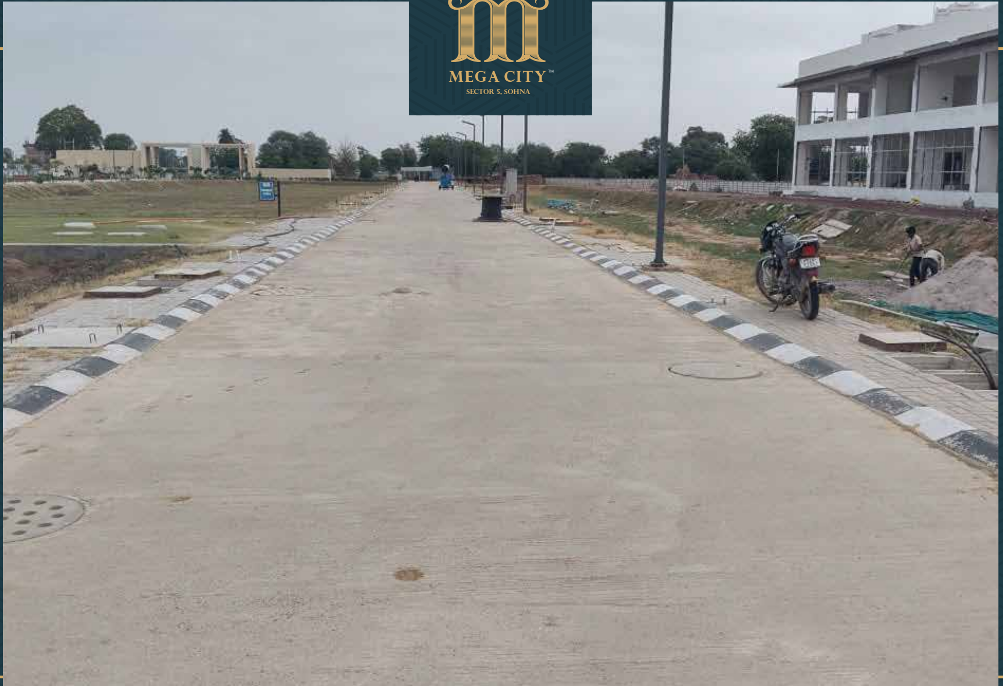
Road no. 5 development work completed including electrical cable lines. Plantation work in progress.
