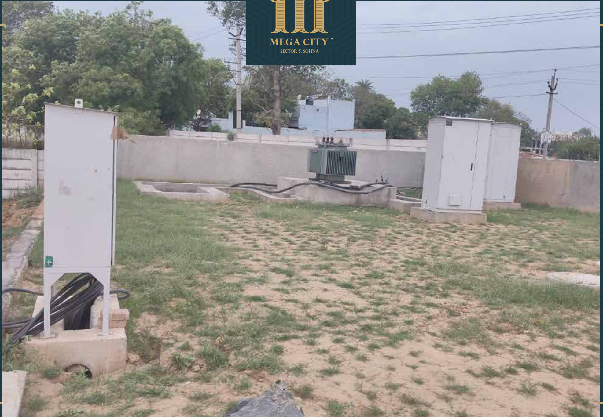
Electrical sub station 2 equipment installation done
