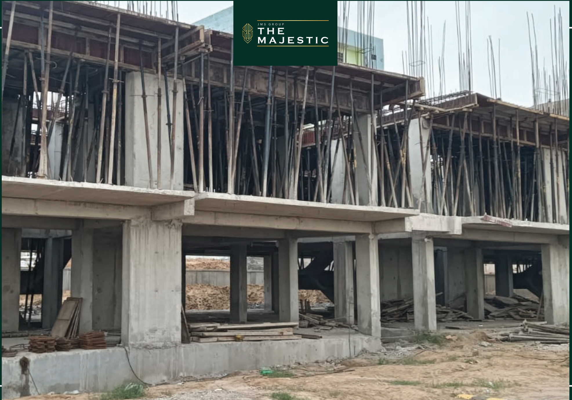
Plot no. 369-373 2nd floor steel and electrical conduit fixing work in progress
